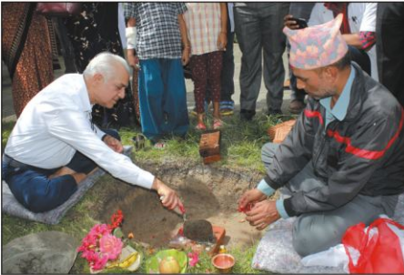
Stone foundation for new CSSD building for Chair Prof. Dr. Ashok Kumar Banskota
